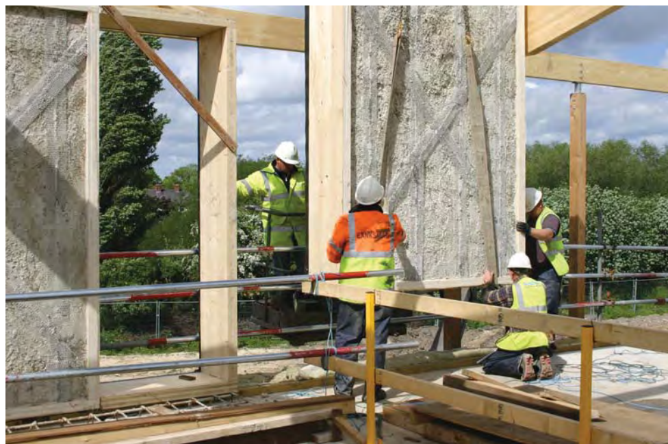
Prefabricated hemp panels being lowered into position – the new extensions could be constructed off site in a similar way
